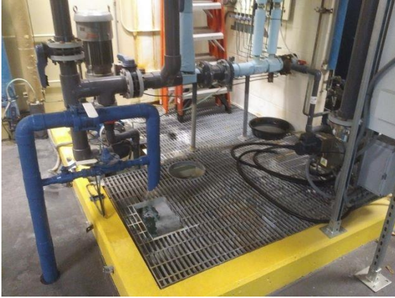
Main Pool Filter
